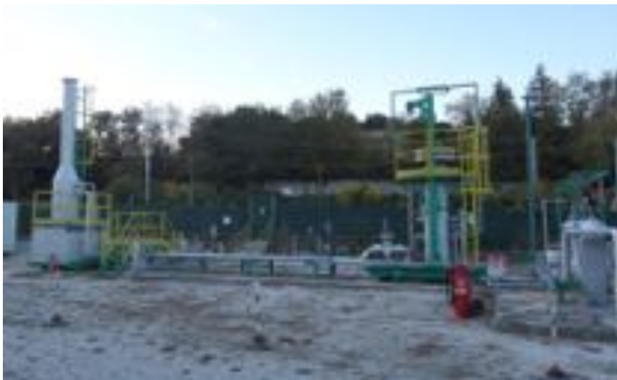
Figure 20-5 Rapagnano gas processing facilities (Source CGG)
