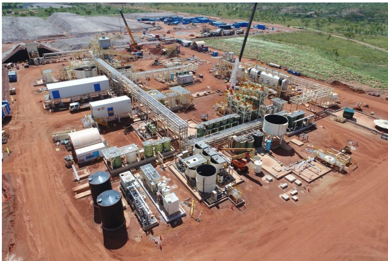
Browns Range Pilot Plant Construction at 28 Feb 18 with Product Estimated to be Shipped from Sept 18 Quarter
