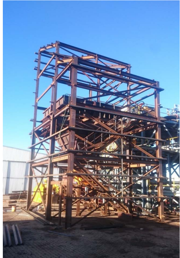
Steelwork for secondary crusher surge bin preassembled prior to transport to site
