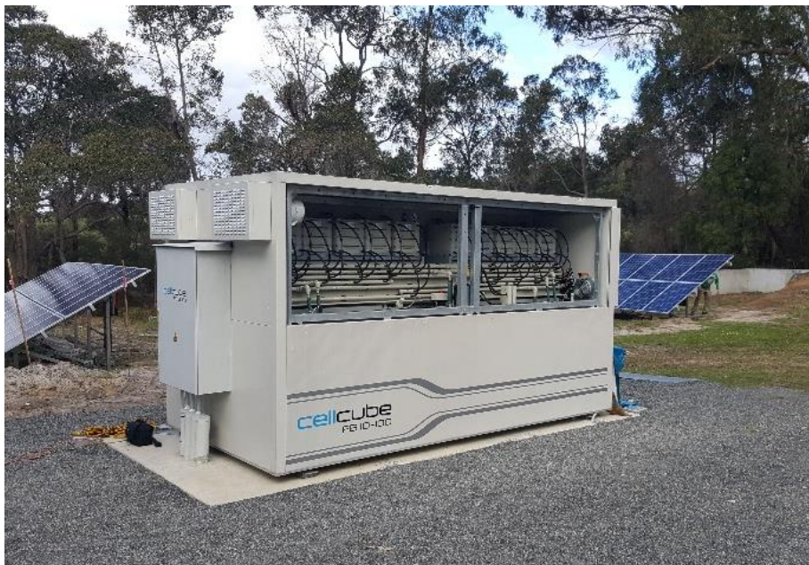
Figure 3 Vanadium redox flow battery in Busselton, Western Australia
