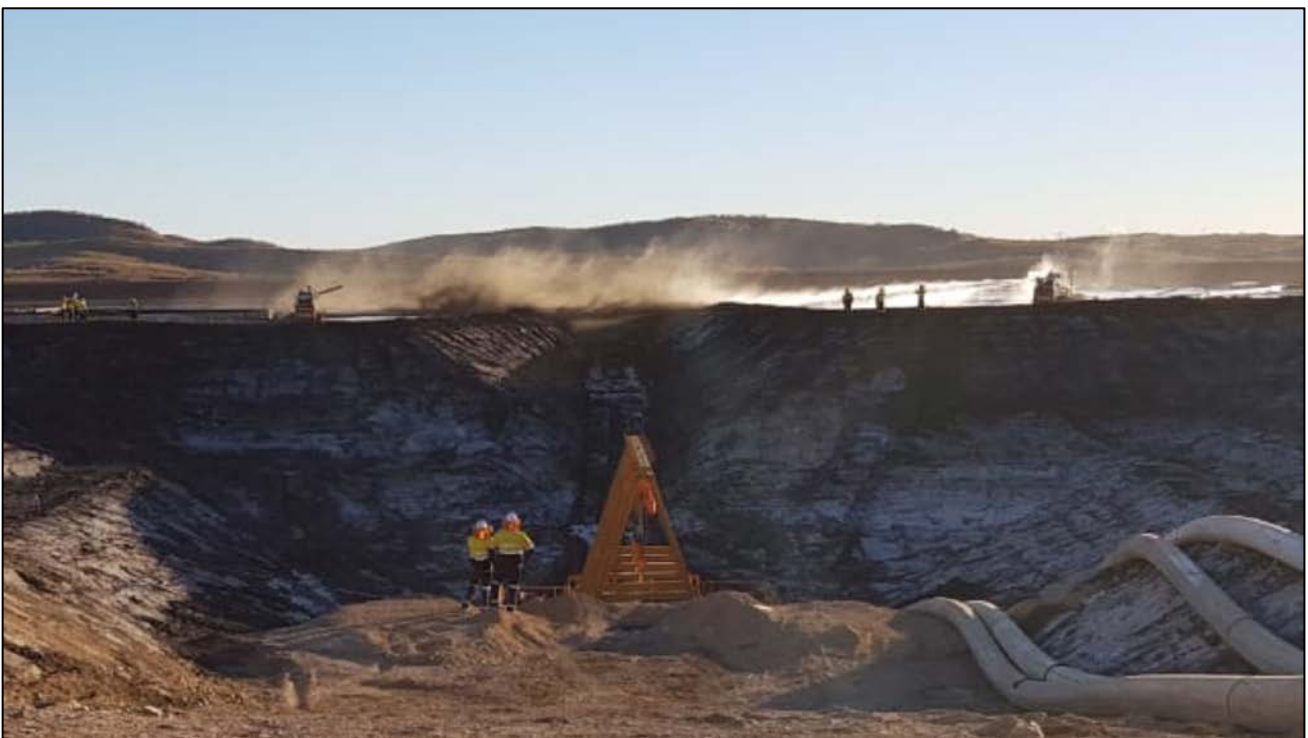
Figure 2: Hydraulic mining of tailings into the Slurry Winning Pontoon
