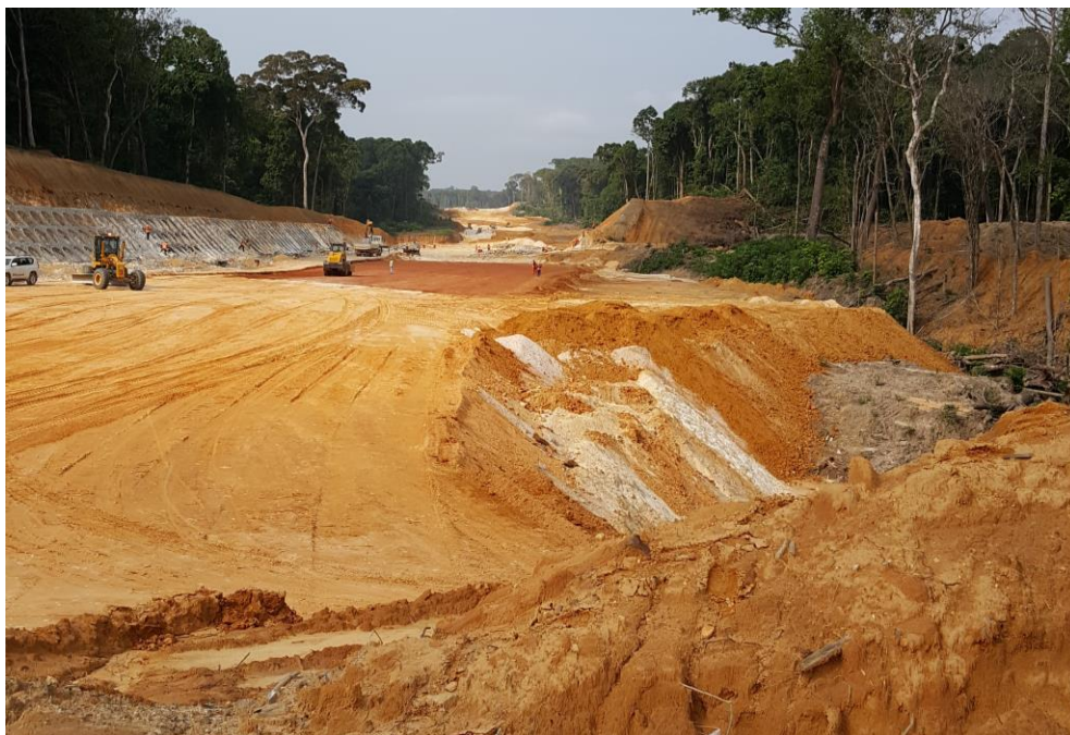
Figure 3: Earth works at the Kribi Port area for the new highway and rail
