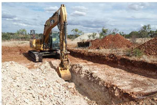
CAPTION: Excavator “free-digging” near surface phosphate rock at Ardmore for bulk samples.
