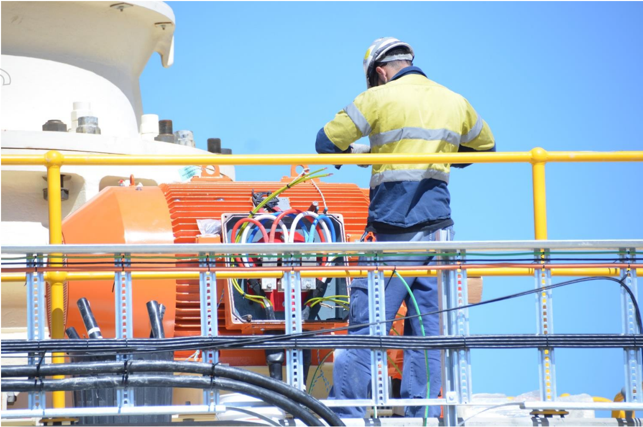
Figure 5: Secondary (cone) crusher electrical connections (13 September 2018)
