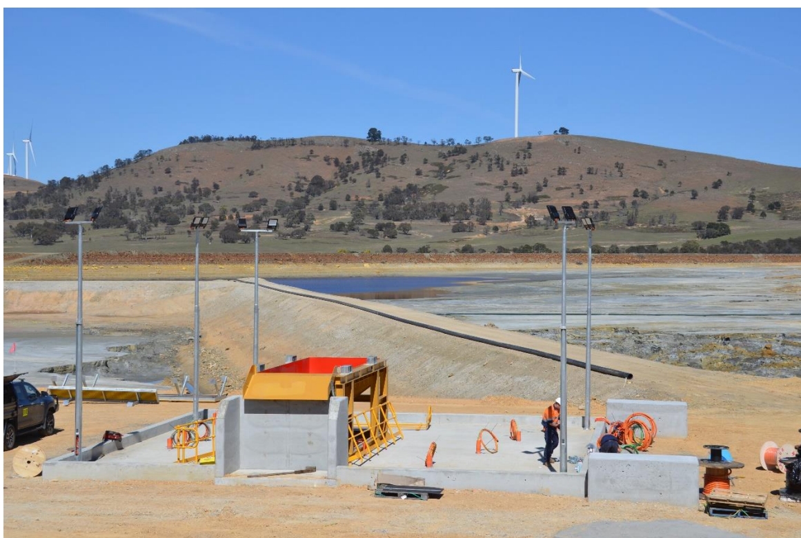
Figure 2: Hydraulic mining infrastructure – pump foundations and trash screen substrate (13 September 2018)
