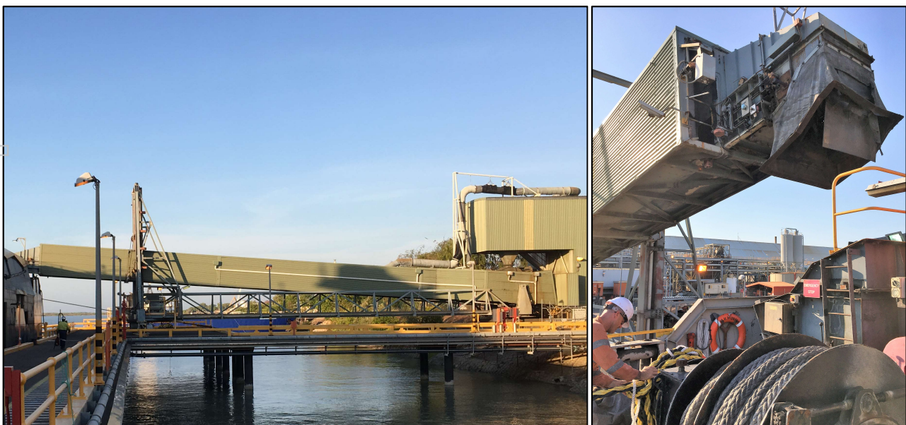
Figures 1 & 2: Karumba Port ship loading conveyer being positioned for concentrate loading onto the MV Wunma
