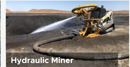
Hydro Mining Ops Centre
