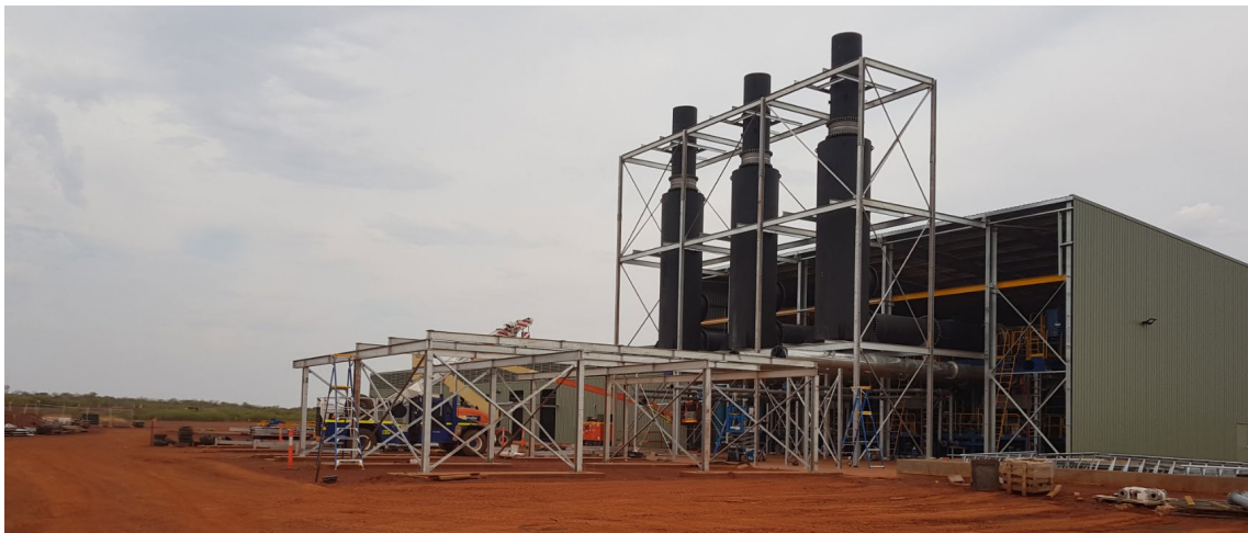
Dead Bullock Soak Power Station exhaust system under construction at Newmont Mining Corporation’s Tanami Operation.
