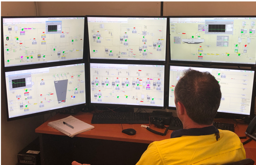
Boonanarring Project Wet Concentration Plant Control Room
