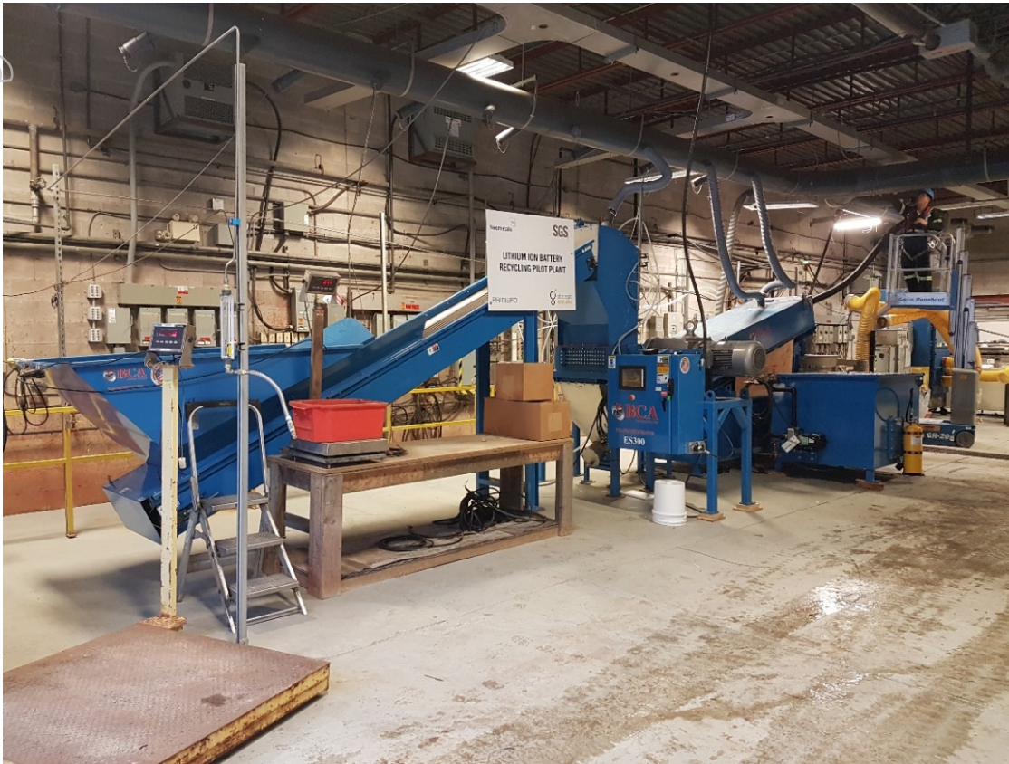
Image 2 – Stage 1 feed preparation plant ready for pilot commissioning in Canada
