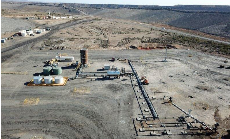
LCEP Syngas Facility
