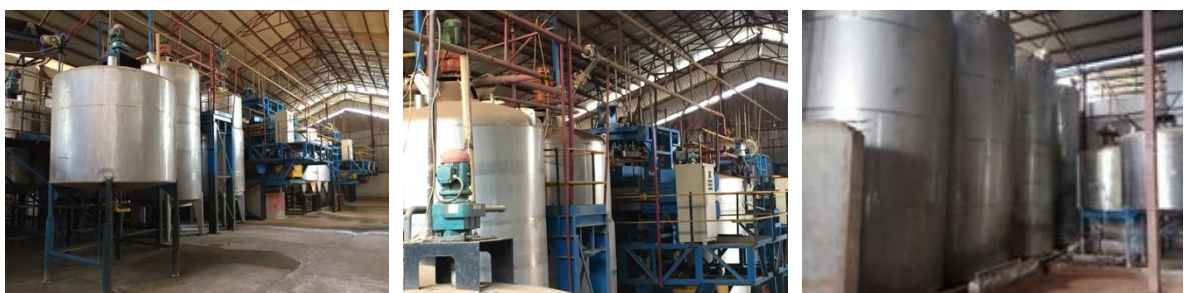
Figure 10, 11 and 12: The Luapula Processing Facility Precipitation Section
