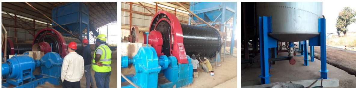
Figure 4, 5 and 6: The Luapula Processing Facility Milling and Slurry Storage Sections
