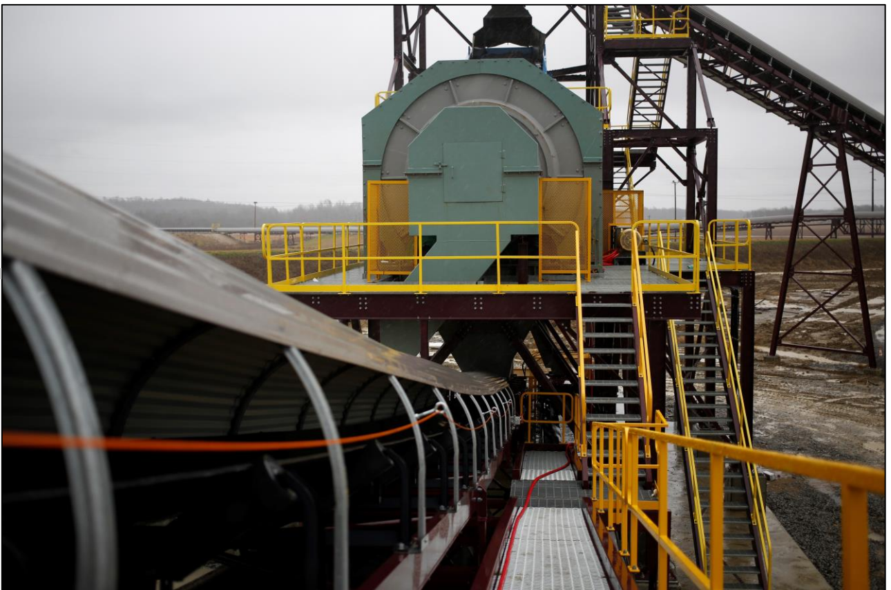
Figure 4: Rotary breaker feeding raw coal to the Poplar Gove CHPP
