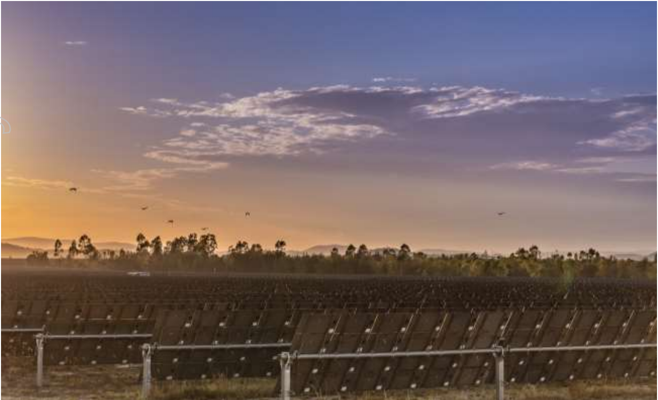
Figure 1. 50MW Kidston Solar Project.
