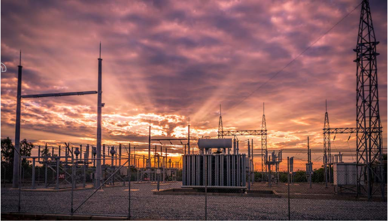
Figure 1. Kidston substation, North Queensland.
