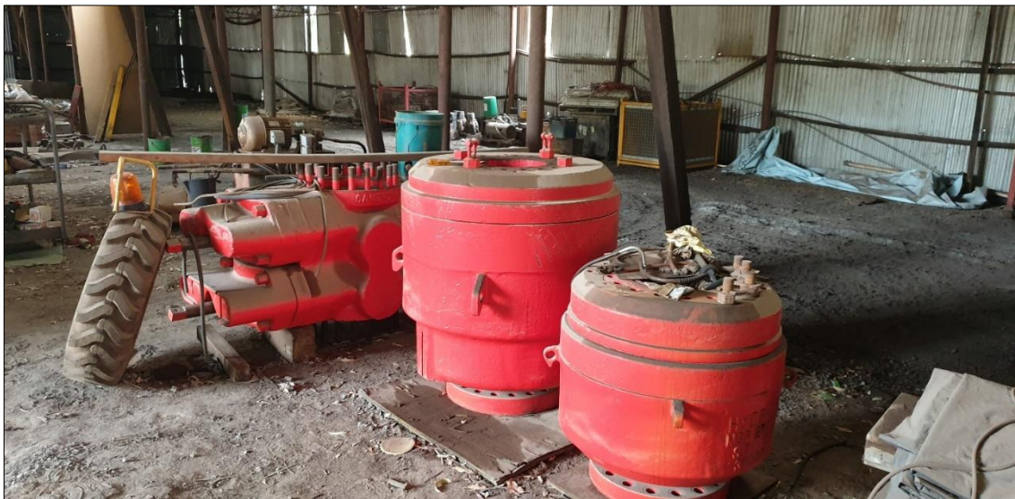
Inspection of larger pipe and blind rams and the large and small hydril components of the BOP (April 2019)
