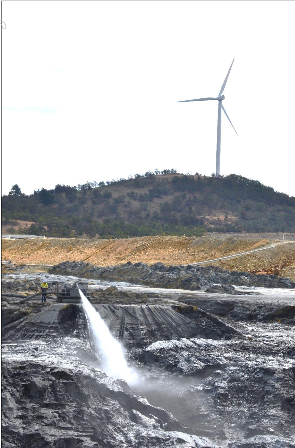
Figure 3 Establishing the production channel at Tailings Dam South during hydraulic mining operations.
