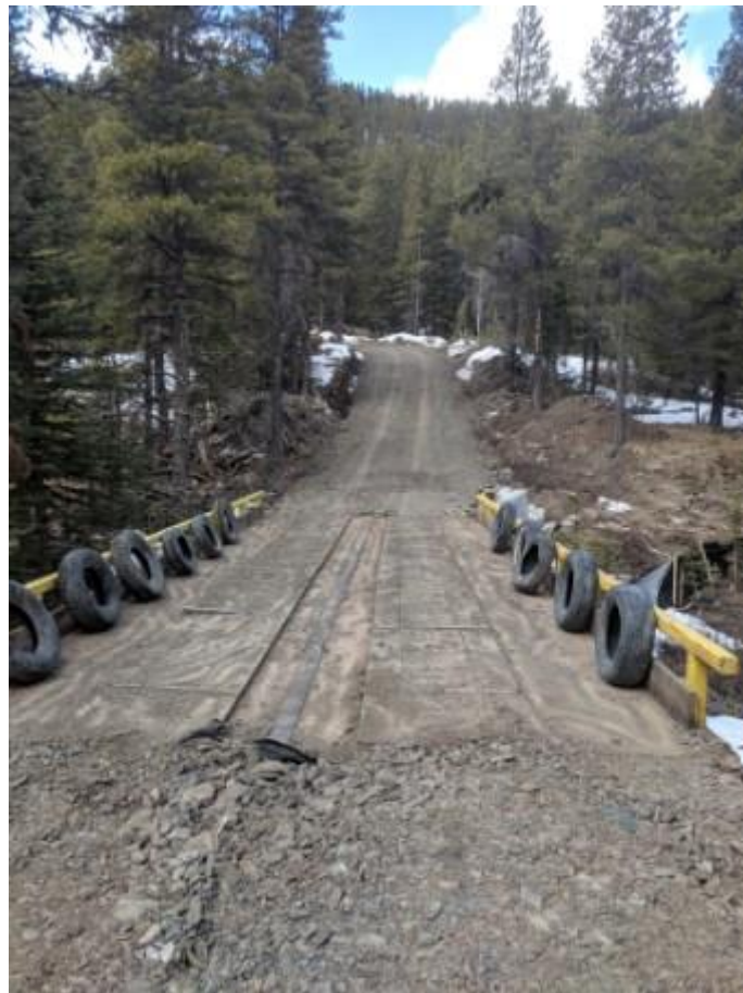
Figure 1. Rehabilitation of access roads to drilling and environmental monitoring sites during 1Q 2019
