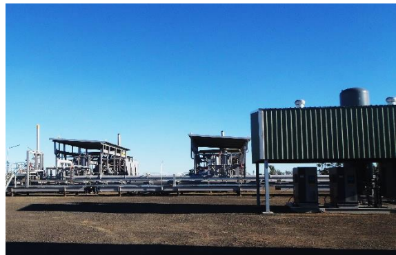
Compression equipment and pipe rack
