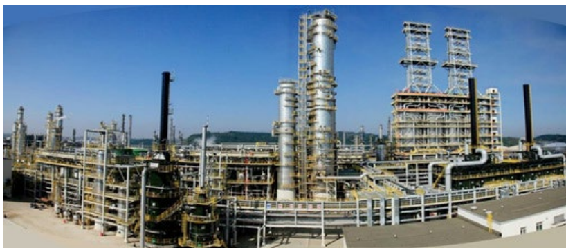
CNE fertiliser plant
