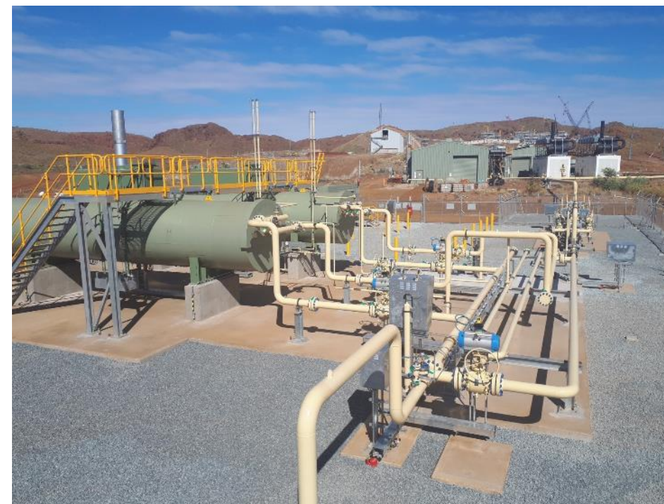
Wodgina Gas Pipeline Delivery Station
