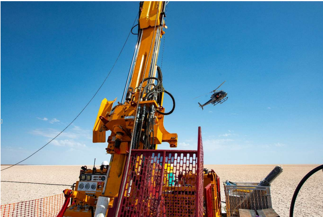
Photo 2: Lake Torrens drilling is helicopter supported to avoid heavy vehicle traffic on the salt lake crust, January 2019
