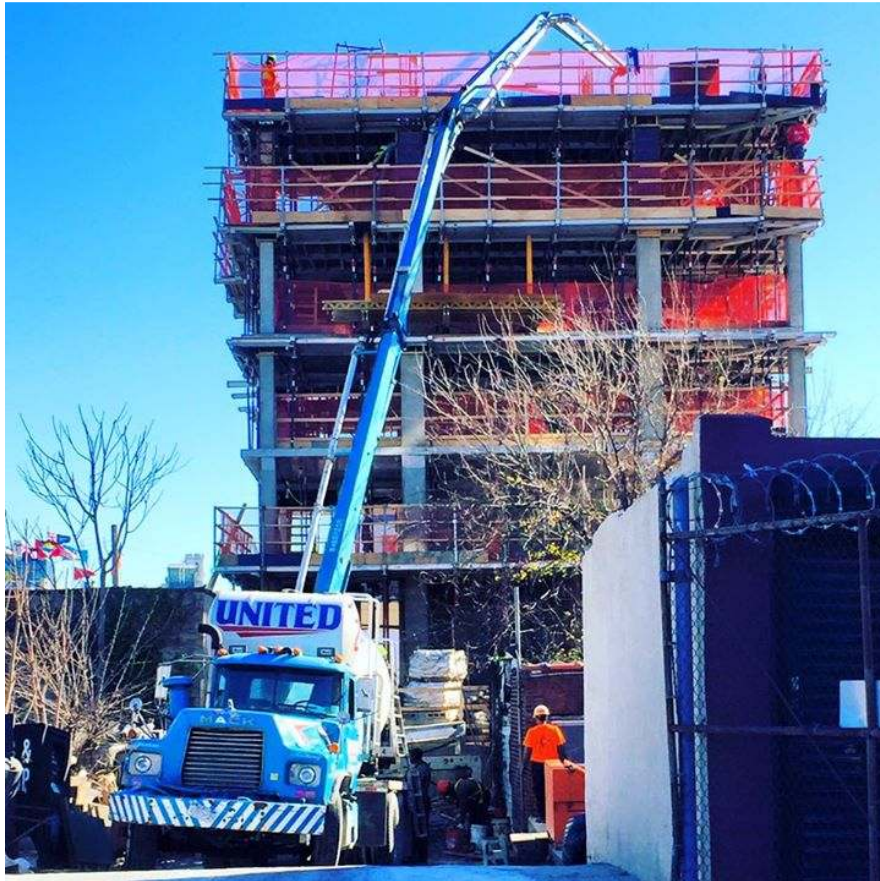
Figure 2. United Transit concrete being supplied to a construction project in New York
