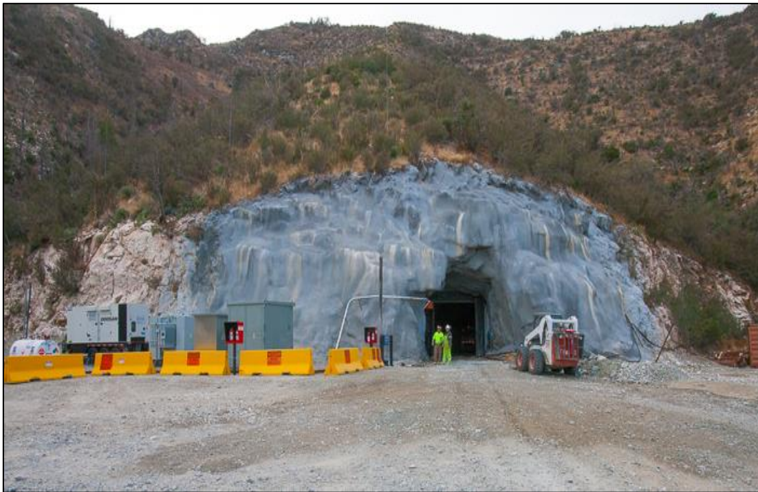
Figure 10 Refurbished 6400 Level portal with electric power infrastructure to left of portal. Note that generator shown in this photograph is currently off site
