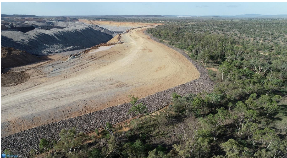
Figure 3: Isaac Plains levee bank alongside Smoky Creek – similar construction required at Isaac Downs alongside the Isaac River
