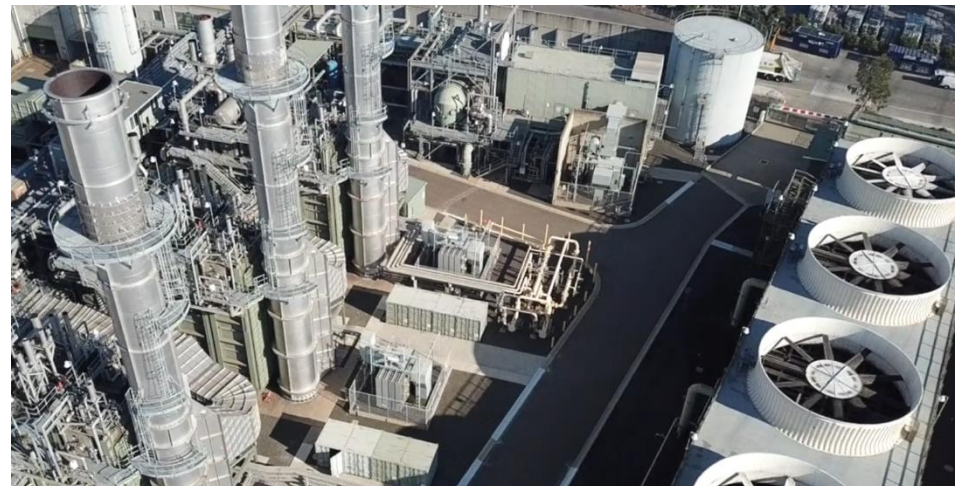
Smithfield Open Cycle Gas Turbine, NSW
