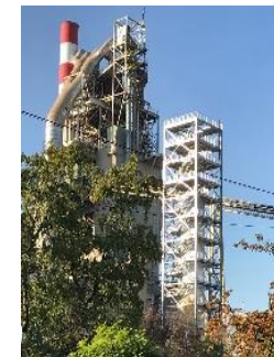
Project LEILAC 1, Belgium
