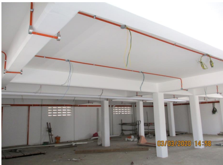
Figure 5 – Electrical substation internal detailing March 2020
