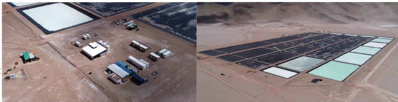
Figure 1: Completion of pilot plant construction (left) and over 30% of pilot pond were filled with brine (right) at the end of the quarter
