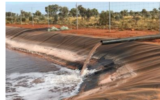
Image: Typical HDPE lined Water Pond
