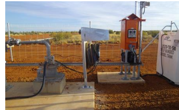
Image: Typical Bore Field Pump Station
