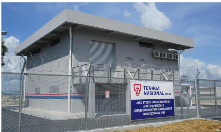
Figure 1: Completed electrical substation, Altech HPA plant site
