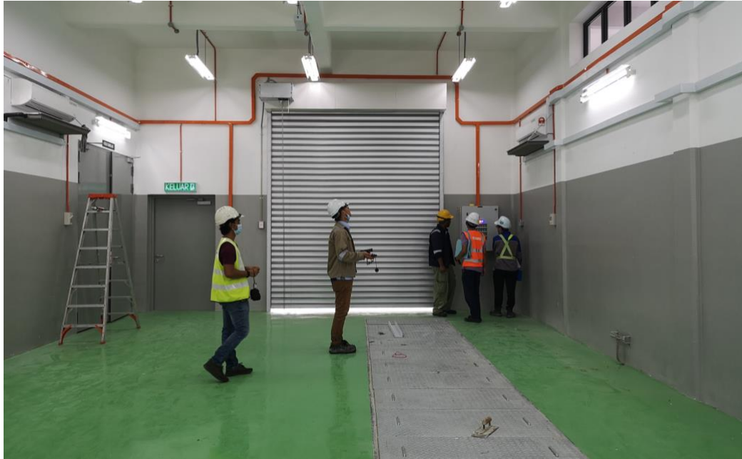
Figure 4: Substation Inspection and Function Checks
