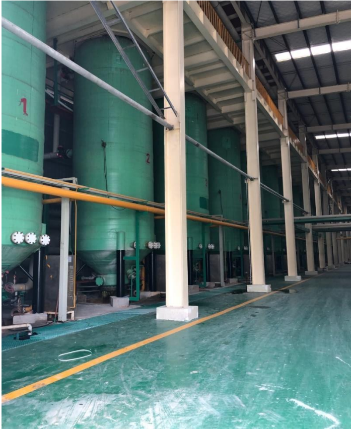
Chemical pickling vats
