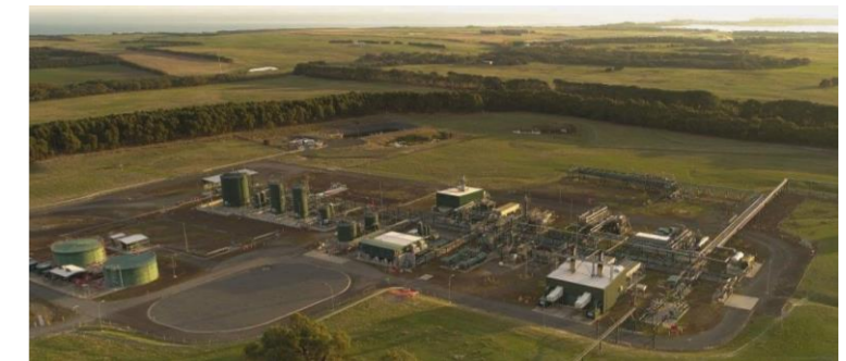
Athena Gas Plant, Onshore Otway
