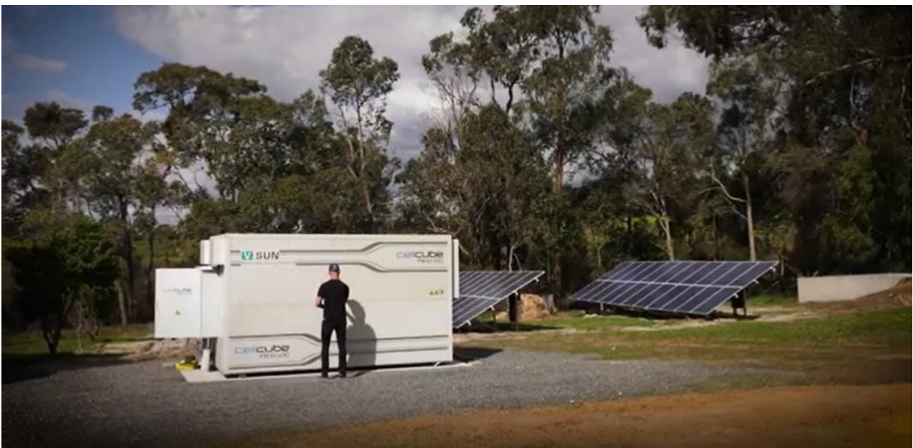
Figure 3 Installing a 10kW/100kWh VRFB at a native tree nursery in Busselton, Western Australia
