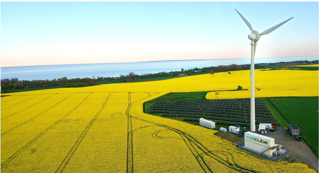
Figure 2 Solar, wind and VRFB installation © Enerox
