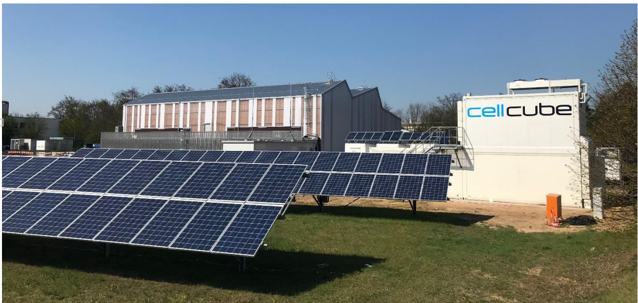
Figure 1 Solar and CellCube VRFB installation at a commercial and industrial site © Enerox
