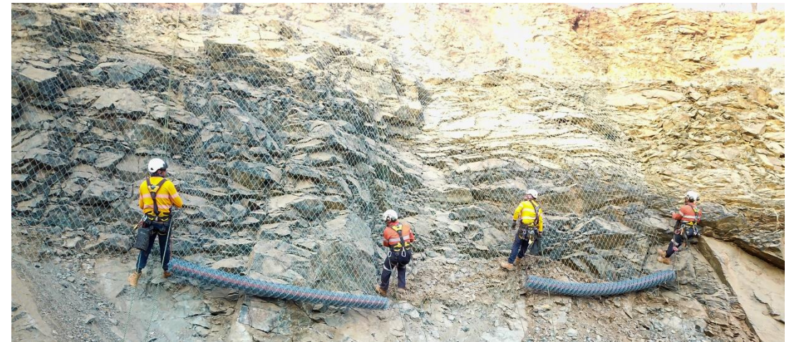
Ground support securing Paris Pit wall face above and around the new portal 24
