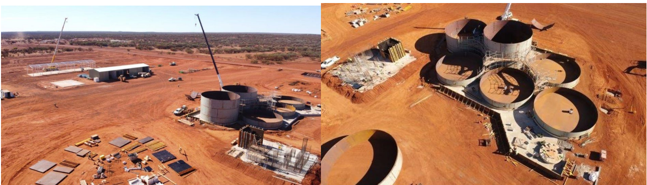
Figure 3: Processing plant construction progress and concrete foundations for the ball mill and CIL tank construction
