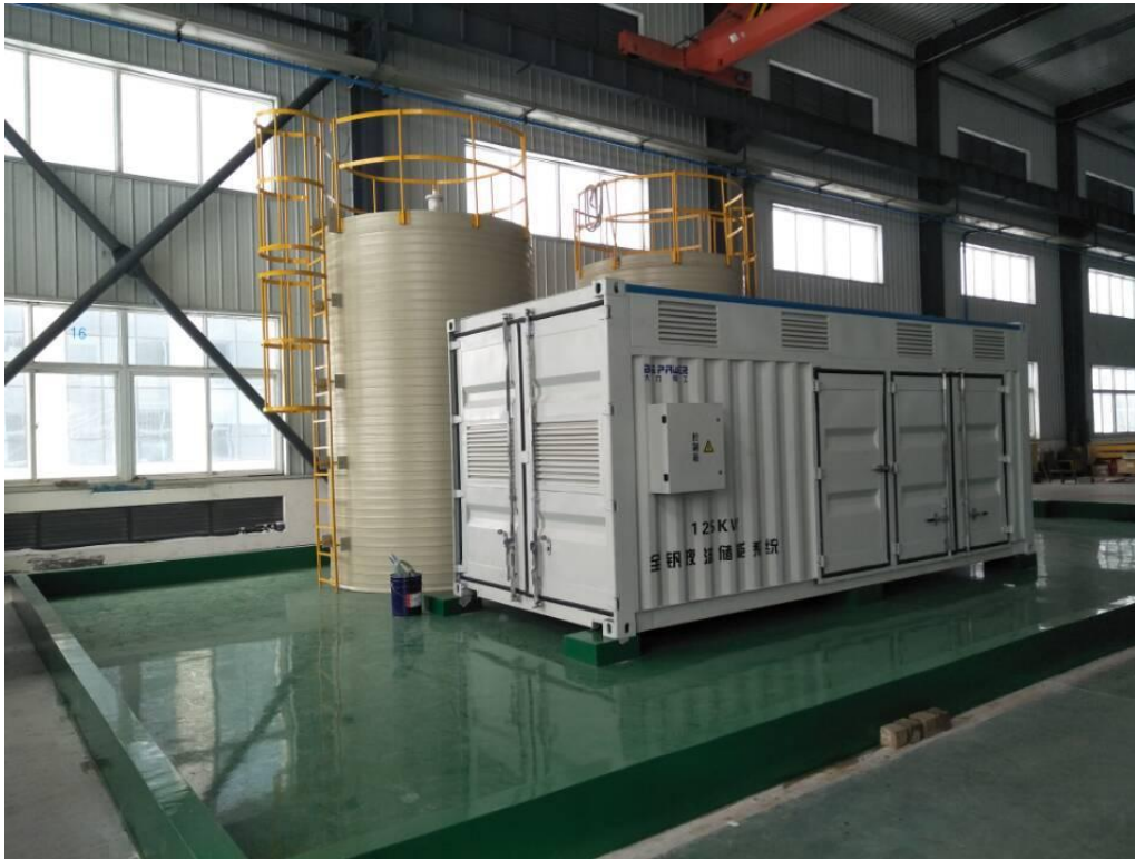
Figure 3: Big Power VRFB System at Xiangyang Used for Peak Shifting
