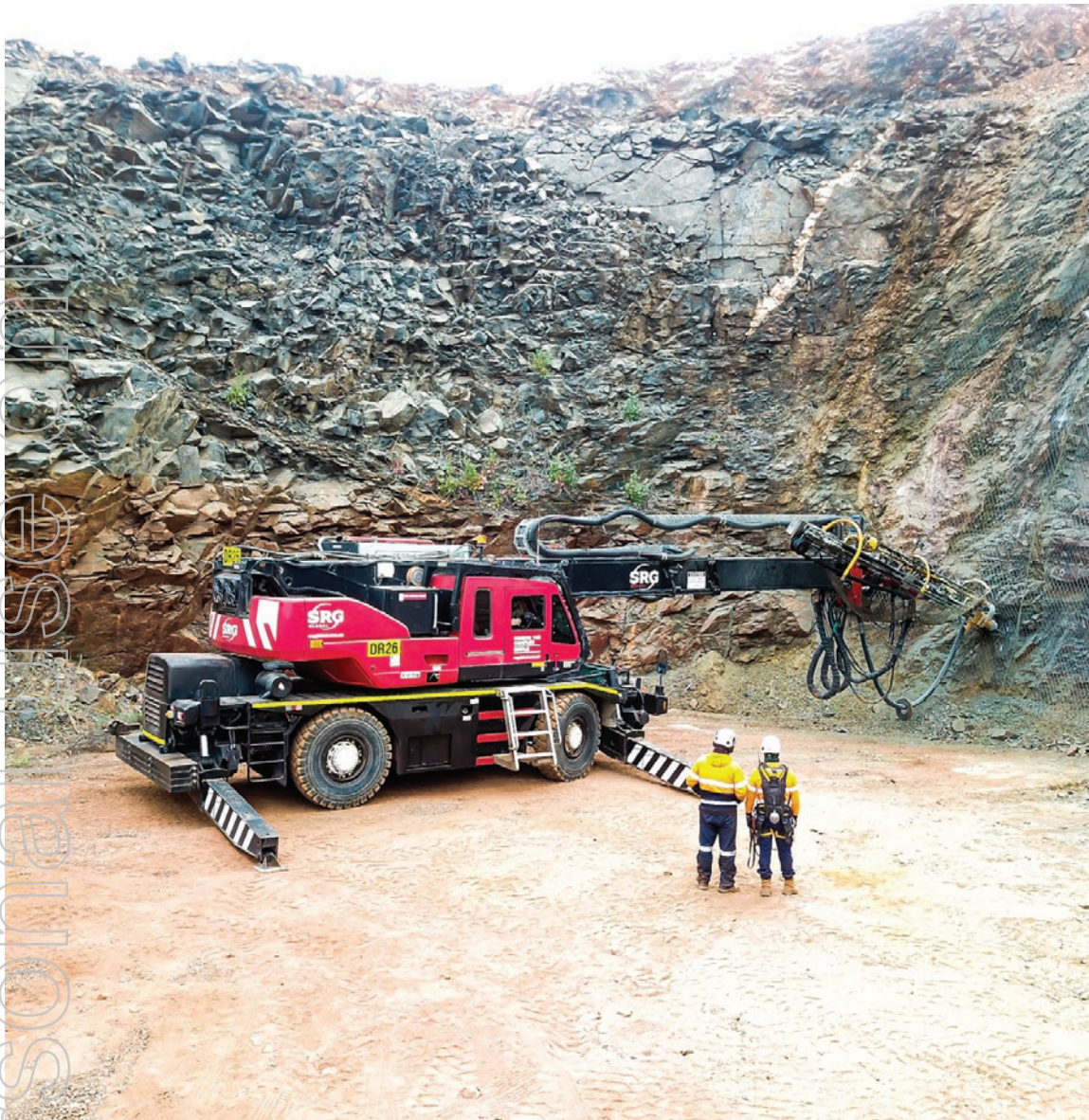
High reach drill in Paris Pit installing ground support for the new portal to be established.
