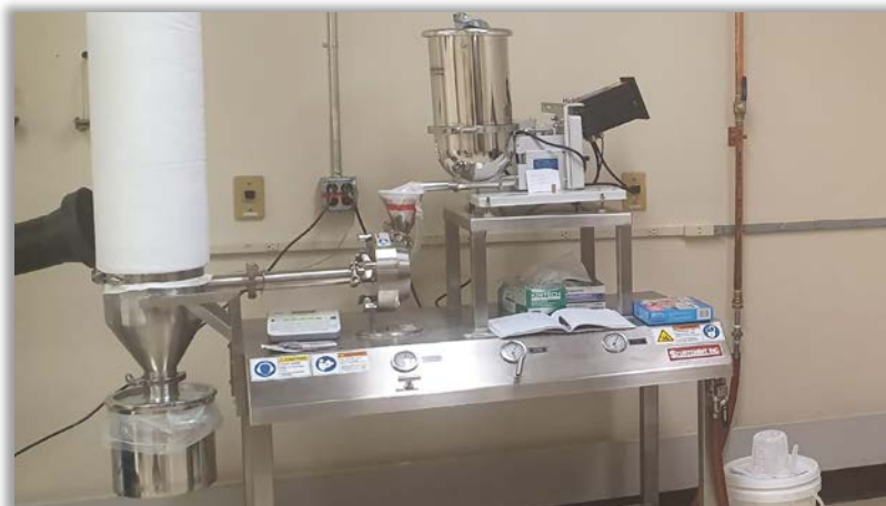
Alpha's dedicated jet mill installation – Binghamton, USA
