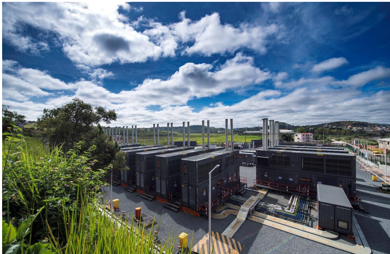
An example of the power solution to be provided by Aggreko.
