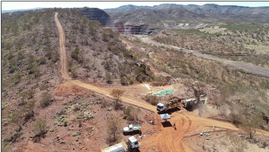
Figure 3: RC drilling at Connie's Find, approximately 400m to the west of the Waugh Pit shown in the background
