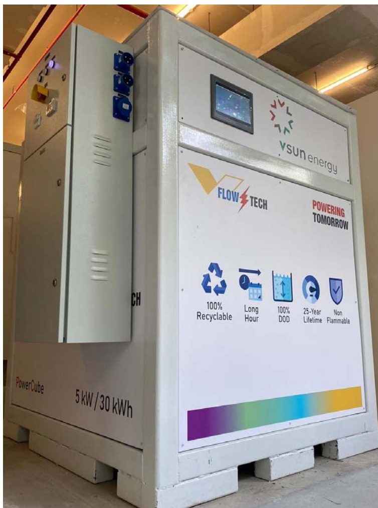
Figure 6 A 5kW/30kWh V-Flow VRFB
