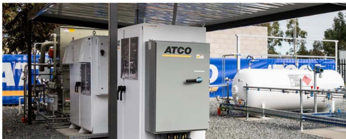
Figure 5 ATCO's Clean Energy Innovation Hub in Jandakot, WA
