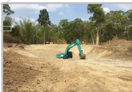
Figure 23 | Process Plant Sediment Pond
