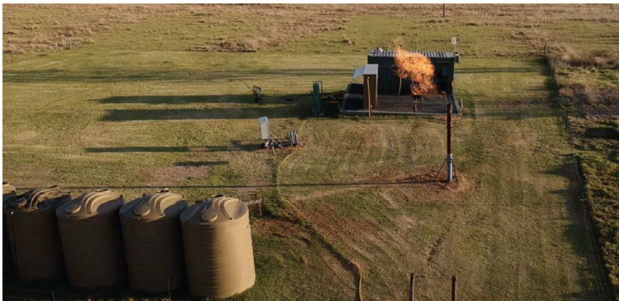
Figure 2 - Pilot production well KA-03PT flaring gas at Amersfoort Project
