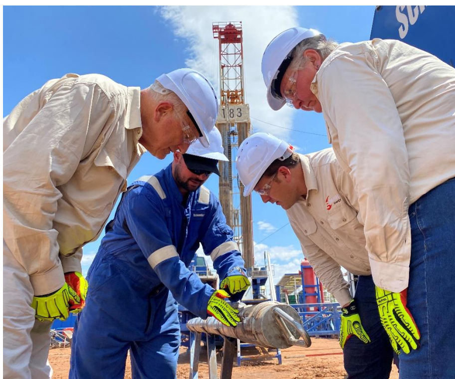
L to R: Chairman Paul Espie, Schlumberger site manager, Managing Director Alex Underwood and NT Senator Sam McMahon at Carpentaria-1 site
