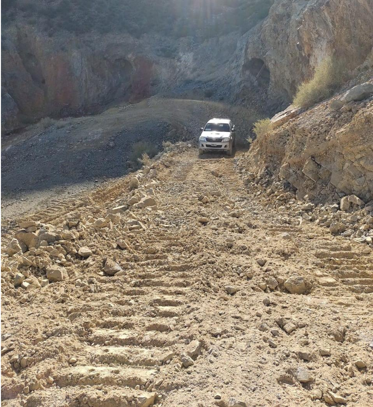
New access road into the Hualilan Hills at Cerro Norte for the man portable drill rig to test the bonanza zone
