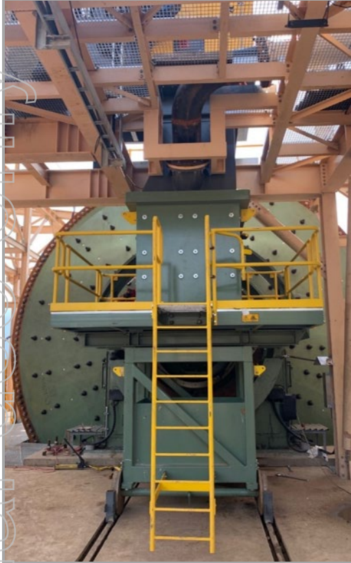
Figure 10 | SAG Mill – commissioned and operating
